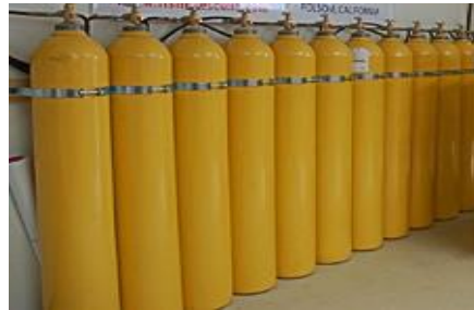
5500 cubic feet of Hyper-clean modified grade E air storage.
